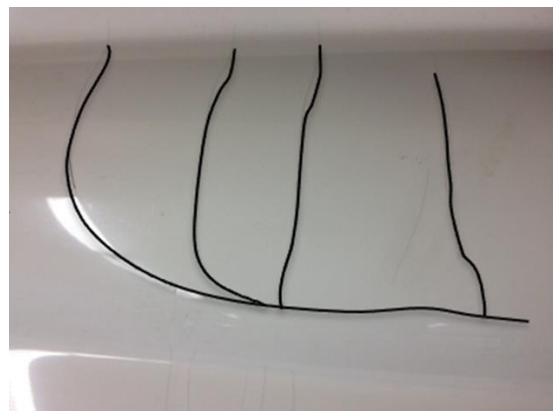
Highlighted zone of gelcoat cracking.
